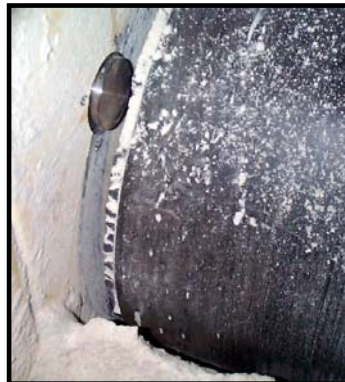
Enclosed Belt Conveyor Application
